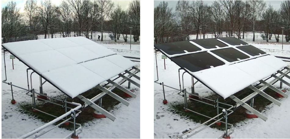
Figure 14: Snow melting (bottom modules disconnected | 14 Feb. 2025 | Ottendorf-Okrilla)
