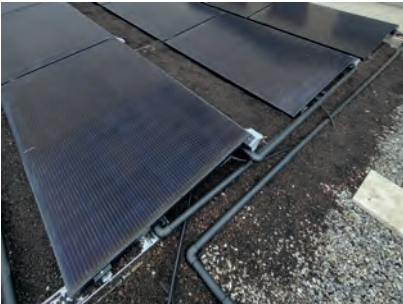
Private pool heating, Switzerland
